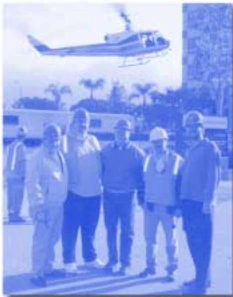
The crew of the Operating Engineers Trust Funds building at 301 N. Lake Ave. prepares to replace a 325-ton chiller with help from a helicopter.
